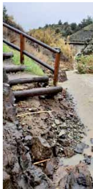
The destroyed old wooden structures. Photo by the Geological Survey Department.
