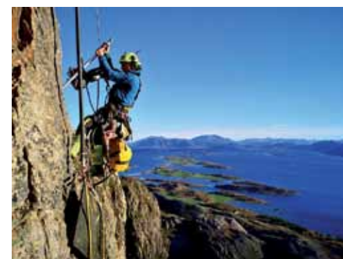
A worker using a pinch point bar to remove loose rocks from the rock face.
